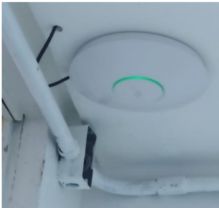
Figura 22 - Access Point Unifi UAP
